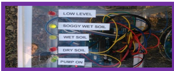
Figure 3.5.3 The soil condition is soggy
